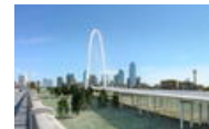
The Margaret Hunt Hill Bridge is now under construction in Dallas. Margaret Hunt Hill Bridge
